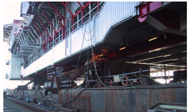
Fig 1 Blast and fire rated escape tunnel on offshore platform (Photo: Natabelle Technology & Booth Industries)
