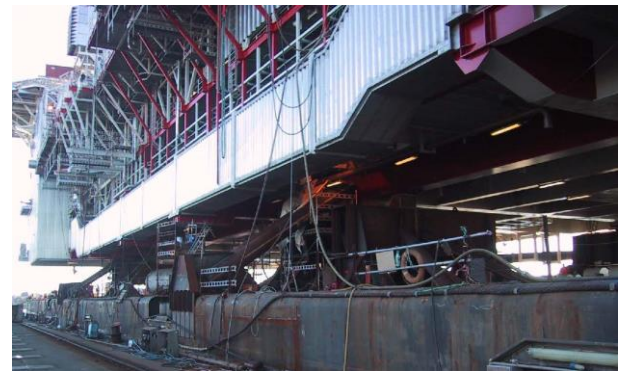
Fig 1 Blast and fire rated escape tunnel on offshore platform (Photo: Natabelle Technology & Booth Industries)
