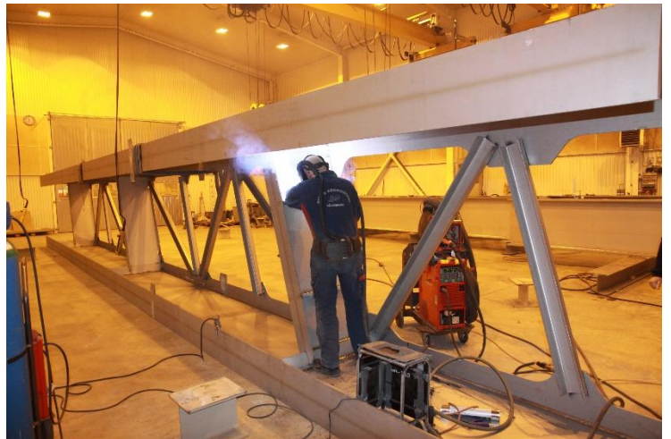
Fig 4 Söderström Rail Bridges fabricated in lengths of 52-75 ft (16-23 m) (Photo: Lars Hamrebjörk)
