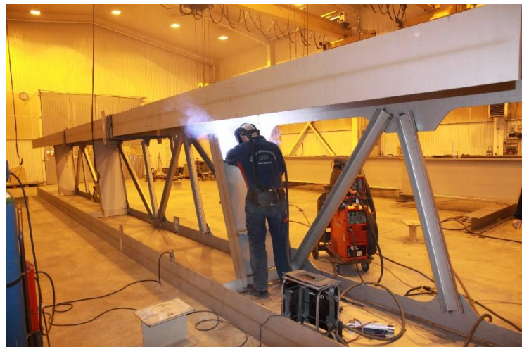
Fig 4 Söderström Rail Bridges being fabricated in lengths of 16-23 m (Photo: Lars Hamrebjörk)
