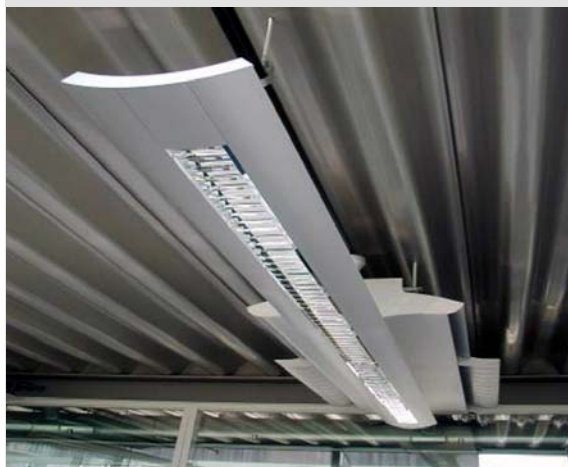
Figure 6: Lighting and air distribution units suspended from the profiled decking
