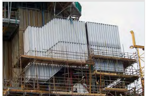
Figure 10: One of the walkway modules connecting the new living modules to the original living quarters
