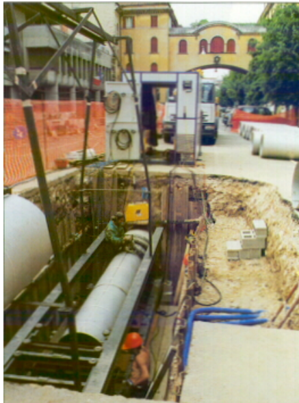
Figure 2. Trenchless relining of a water main in a busy street in Padua, Italy
