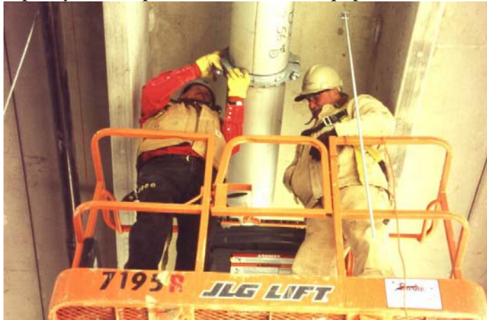
Figure 1. Installation of 300 mm drinking water piping in a sports stadium in Detroit, USA.
