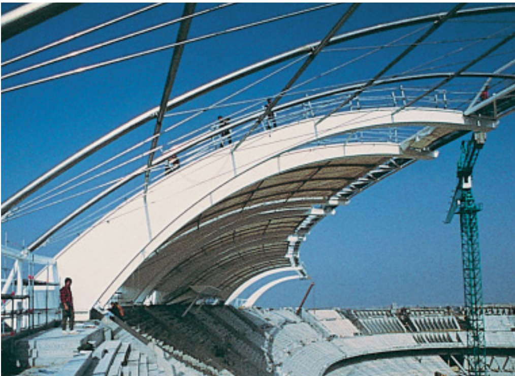
Despite the size and reach of the cantilevered steel girders, the light-permeable roof structure retains a delicate, airy feel.
