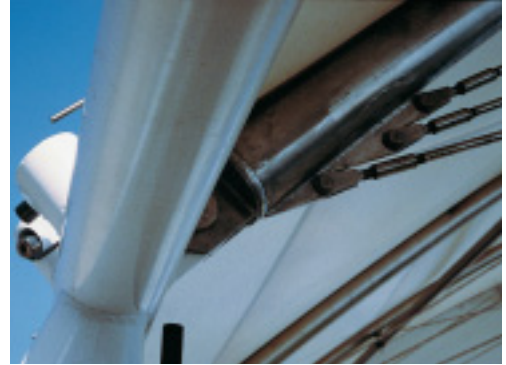
Detail of the connection between the stainless steel tubes and the white-painted steel frame.
