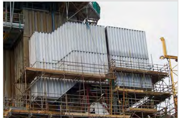
Figure 10: One of the walkway modules connecting the new living modules to the original living quarters
