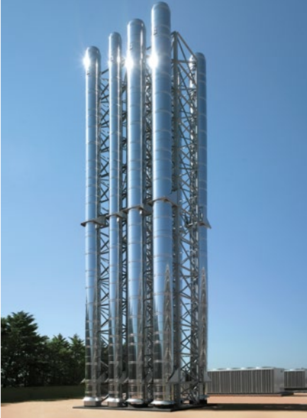
Their combined corrosion and high temperature resistance makes stainless steel an optimal choice for lightweight, elegant chimneys. Photo: Roccheggiani, Camerano, Ancona (I)
