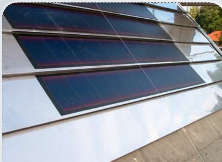
FIGURE 4: Detailed view of the stainless steel tilted roof in Stralsund. Active photovoltaic sections (centre) can easily be combined with non-active ones (right and left).
